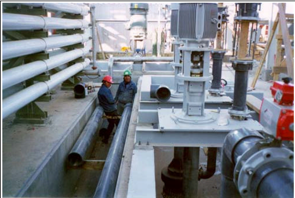
Reverse Osmosis Desalination Facility
