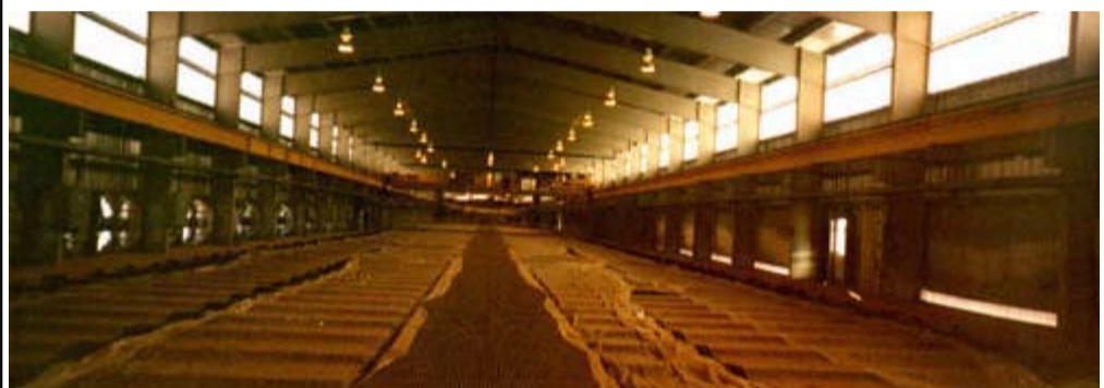
Copper Electrowinning Facility
